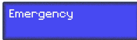
Figure 13.1. Display on LCD screen when emergency stop ON
